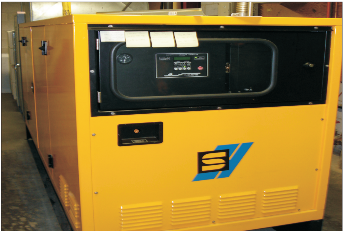
Photograph 2: View of the diesel-fired emergency generator located in the generator room on the first floor.
